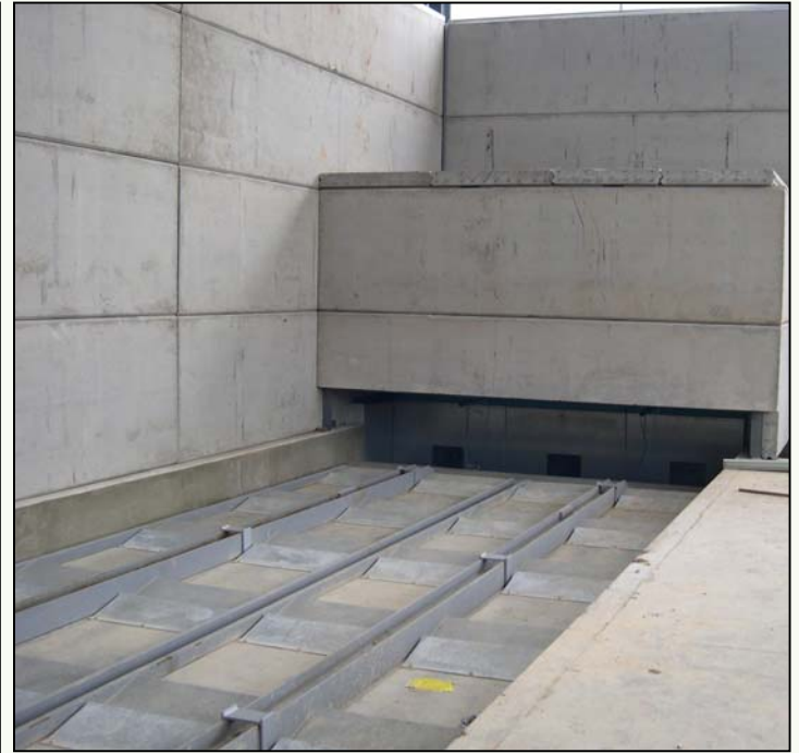
Hydraulic walking floor fuel discharge system
